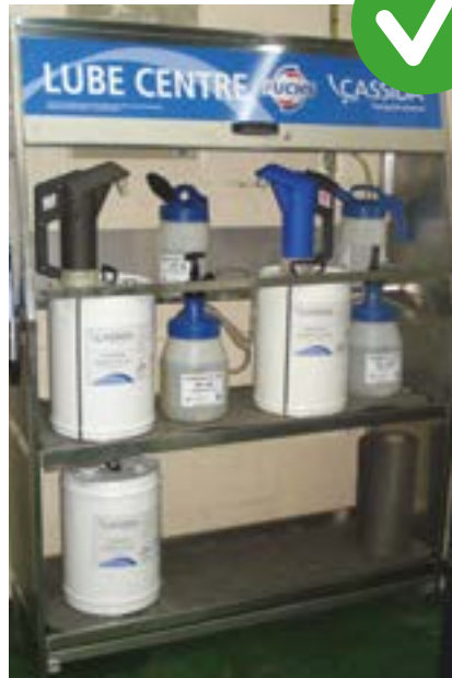
Compliant storage with built-in bund and oil-transfer containers clearly labelled in a clean, designated area
