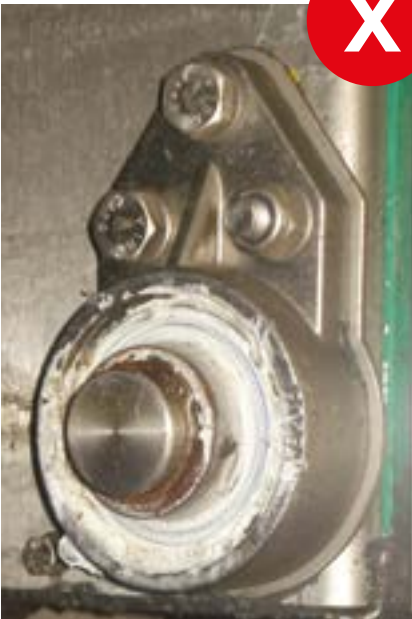
An over-greased bearing is a potential contamination risk. Excess grease should be wiped away to prevent any contaminants adhering to the surface.
