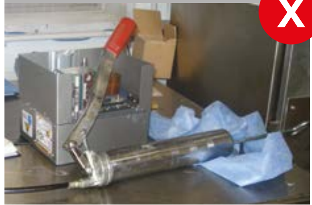
An unmarked grease gun means that it is not known whether food-grade or non-food-grade grease is in use. This could potentially lead to product contamination
